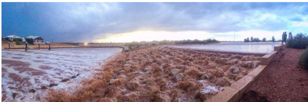
Figure 6-4: Madaffari Drive Spillway in action
