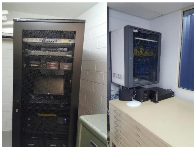
After: Servers now located in a purpose built rack in the Strong Room
