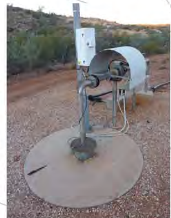
Exmouth Water Supply bore
