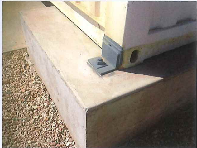
Pictured: A properly secured sea container
