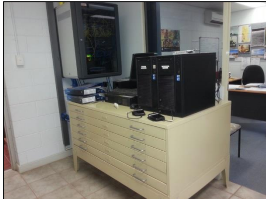
Before: Servers were previously located in Admin General Area
