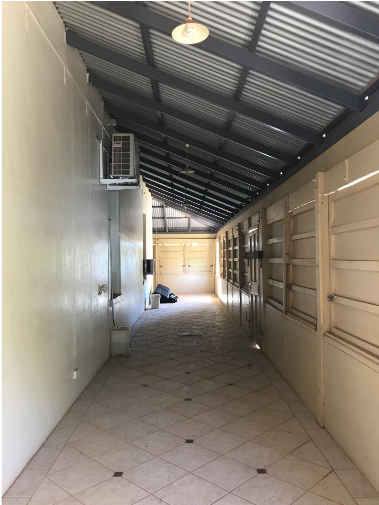
Photograph 8 Typical enclosed verandah. The entire roof was replaced after the loss of the roof in a cyclone. The replacement is steel framed and set a higher level than the original. Kerry Hill Architects, September 2019
