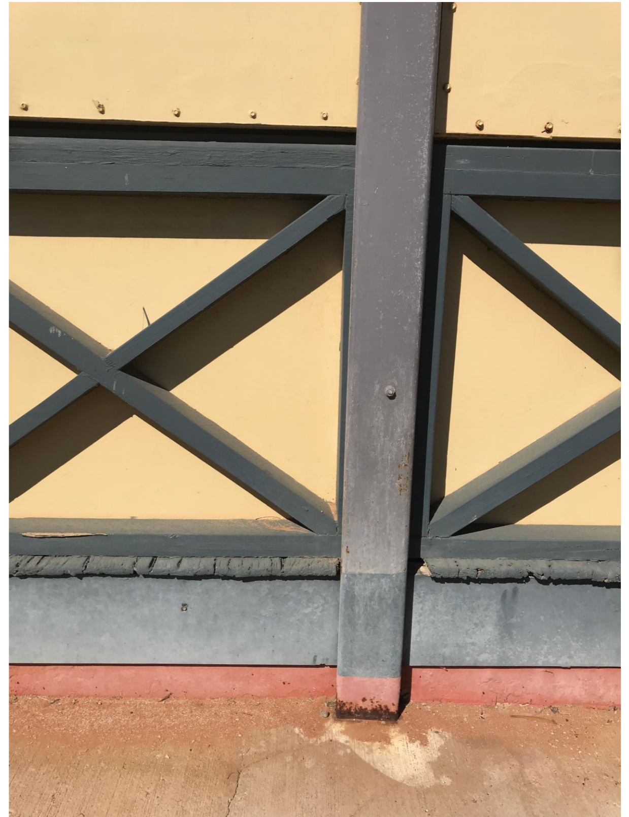
Photograph 5 Steel channels fixed to existing timber posts. Note corrosion to base of the steel and deterioration of the floorboard ends. Kerry Hill Architects, September 2019
