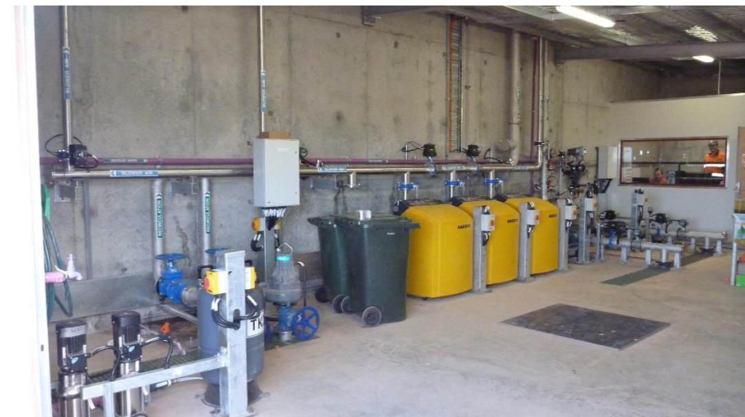
Figure 2 – Monkey Mia Dolphin Resort equipment room
