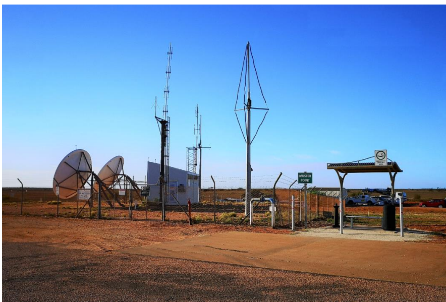
Figure 8 Airservices Australia Satellite Ground Station
